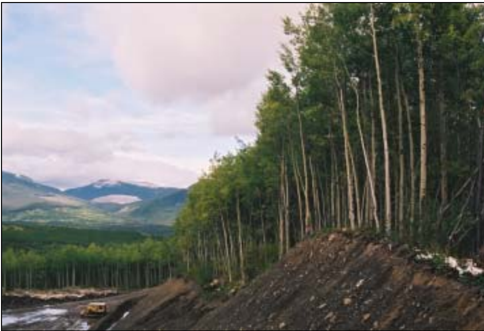
A92. Eastern edge of b-3-G lease facing Station 5, note a few aspen in the foreground have minor mechanical injury to their lower stems.
