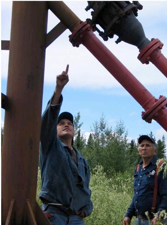
Infractions at Anadarko Well Site near Prophet River
