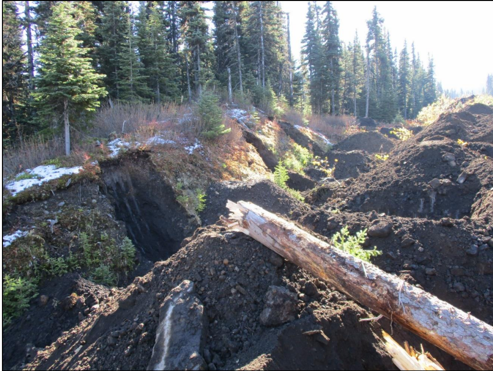
Figure 5. Road deactivation and mounding on the Bickford Mtn.-Fisher Creek FSR site, Klinse-Za Caribou Habitat Restoration Program.
