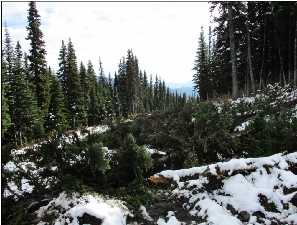
Figure 7. Tree felling across the Bickford Mtn.-Fisher Creek FSR site, Klinse-Za Caribou Habitat Restoration Program.
