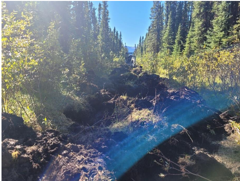
Figure 3 : Mounding on a seismic line after the crew was informed and practiced in the technique. Mounds are across the line with some variation to accommodate for tree and shrub growth along the edges of the seismic line
