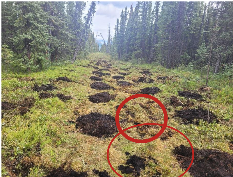
Figure 1: The mounds being excavated when WSP-Golder arrived. Mounds were too small and too far apart to achieve the goals of hindering movement of animals and humans down the seismic line. The red circles shows where the moss layer was being put back into the pits forming a tripping hazard.
