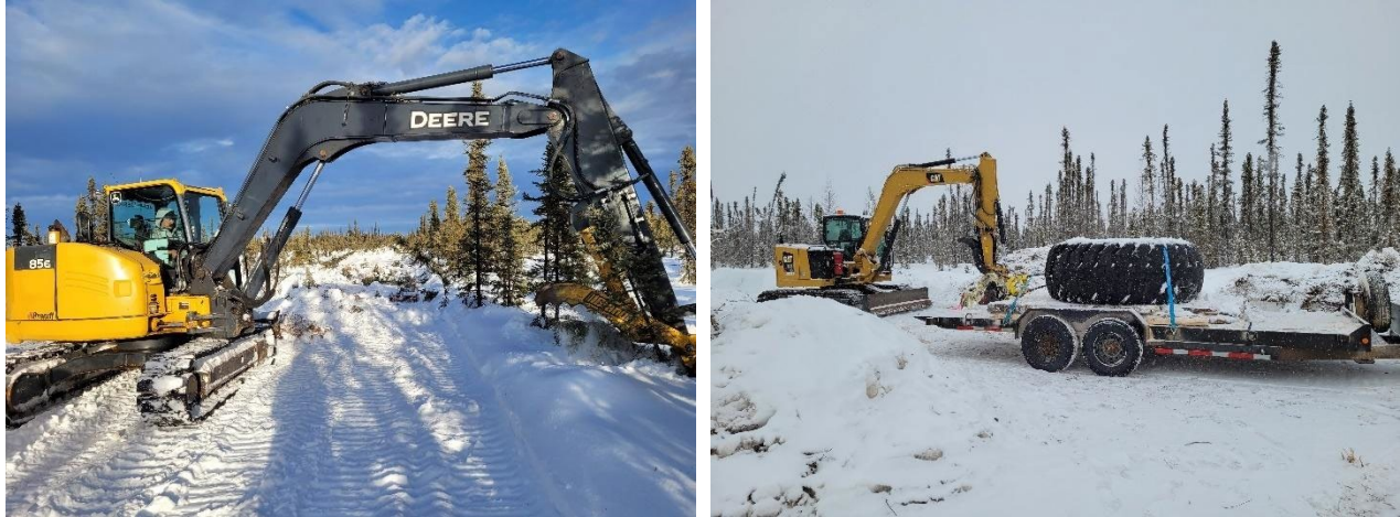
Figure 22. Implementation of restoration during winter 2021-2022 was accomplished using Deere 85G (L) and a Cat 308 (R) excavators. Both machines are smaller mid-sized excavators.
